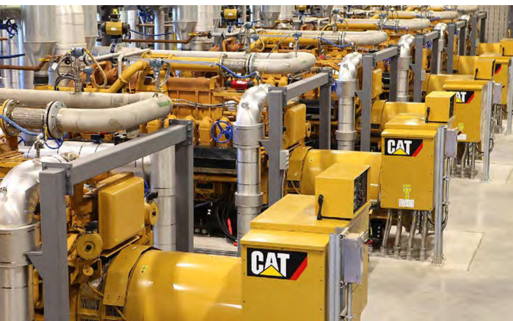
Cat® generator sets installed at a landfill gas processing and power plant near Montreal, Canada, producing electricity from landfill gas.
